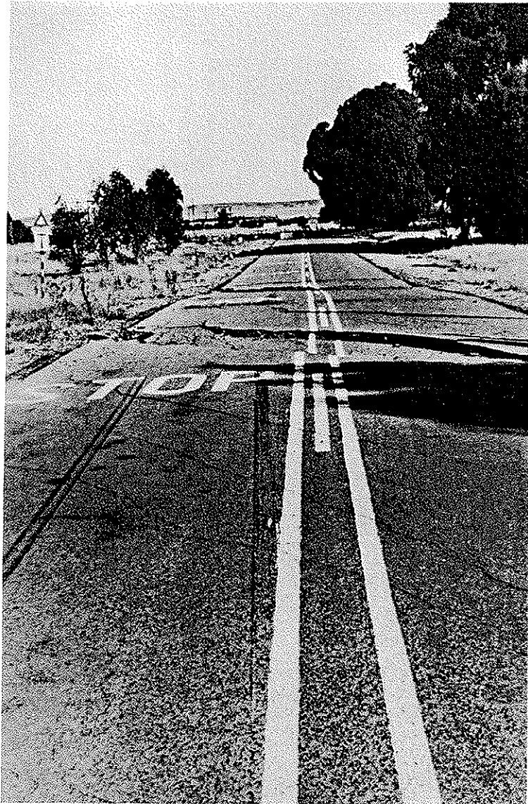
Pl. 4.1 — Cracks in tarmac with vertical and lateral displacement of the road north of Bank Station due to differential subsidence (photo: Geological Survey of South Africa). Barste in teer met vertikale en sydelingse verplasing van die pad noord van Bankstasie weens differensiële saking (foto: Geologiese Opname van Suid-Afrika).
